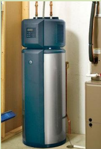
Heat pump water heating unit
