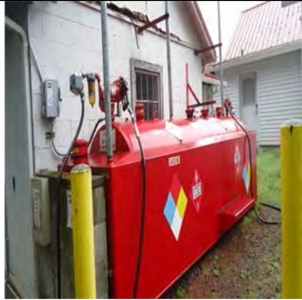
D3011 Oil Supply System.1:- Gasoline and Diesel fuel storage tank
