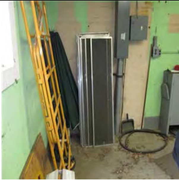
C3012 Wall Finishes to Interior Walls.1:- View of paint finish to CMU walls.
