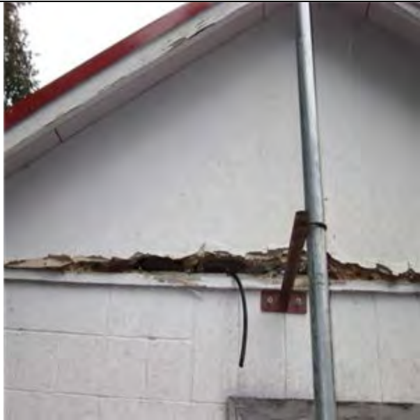
B2011 Exterior Wall Construction.1:- Painted CMU walls and decayed weather board.
