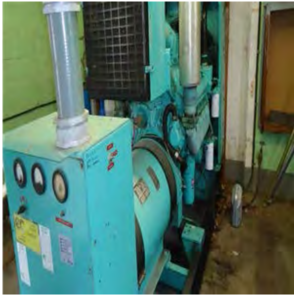
G4092 Site Emergency Power Generation.1:- Generator
