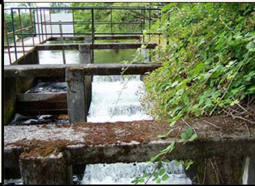
Lower Bennett fish passage facility
