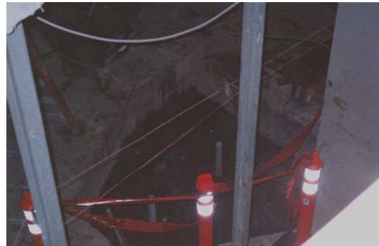
Adding a freight elevator to the State Library. Image of the freight elevator shaft.
