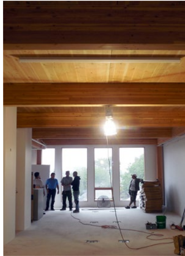
In the Albina Yard building, cross-laminated timber panels were laid horizontally on beams to construct floors between stories. In this photo, the underside or bottom of the panels are viewable as the ceiling.
